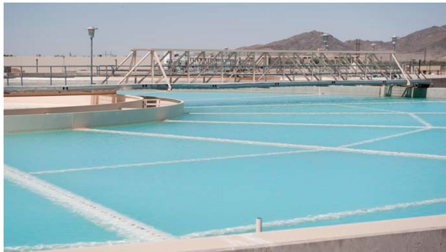
Exterior photo of one of the three large solids contact reactors located on the grounds of the Yuma Desalting Plant. Photo credit: Alex Stephens; Bureau of Reclamation.
