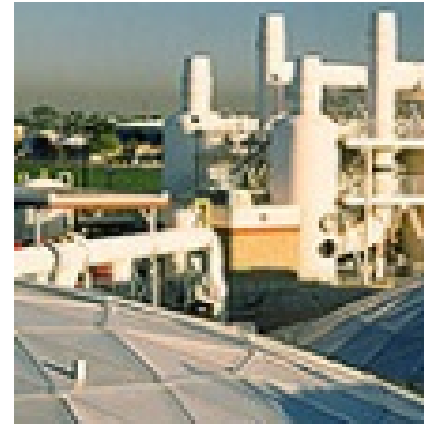
Phoenix 23 rd Avenue Wastewater Treatment Plant
